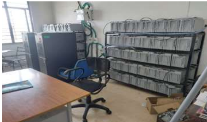
20 KVA UPS to Support Advanced Artificial Intelligence Lab
